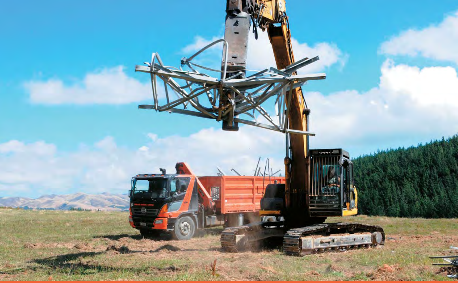
Dismantling decommissioned electricity transmission line pylons has become a Macaulays specialty. Shear attachment on digger cuts the structures into pieces for transporting, while helicopters are sometimes used to lift sub-assemblies to the ground ( opposite page )
