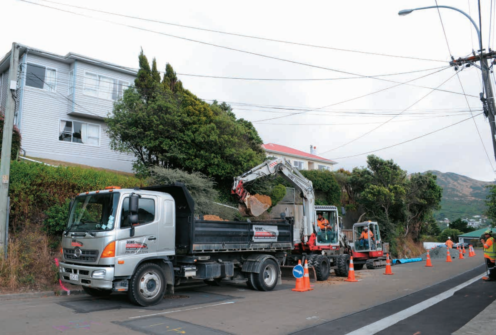
A lot of the company's jobs are on narrow suburban streets, where compact excavators and smaller 4x2 tippers come into their own
